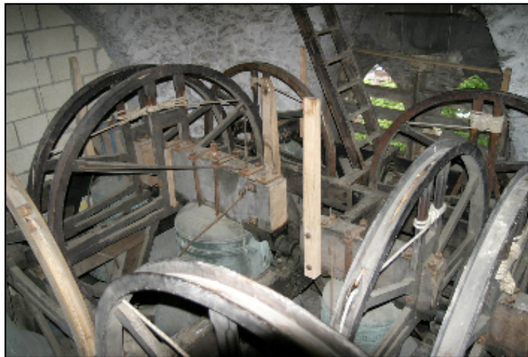
A view of the bell installation. (The 5th wheel is in the foreground)
